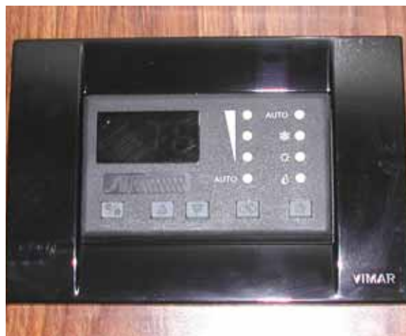
Air Conditioning Control Panel
