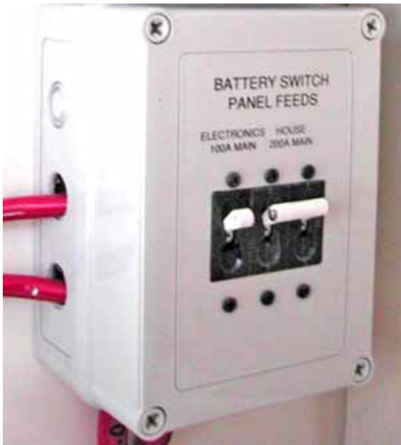
Battery Switch Panel Feeds
