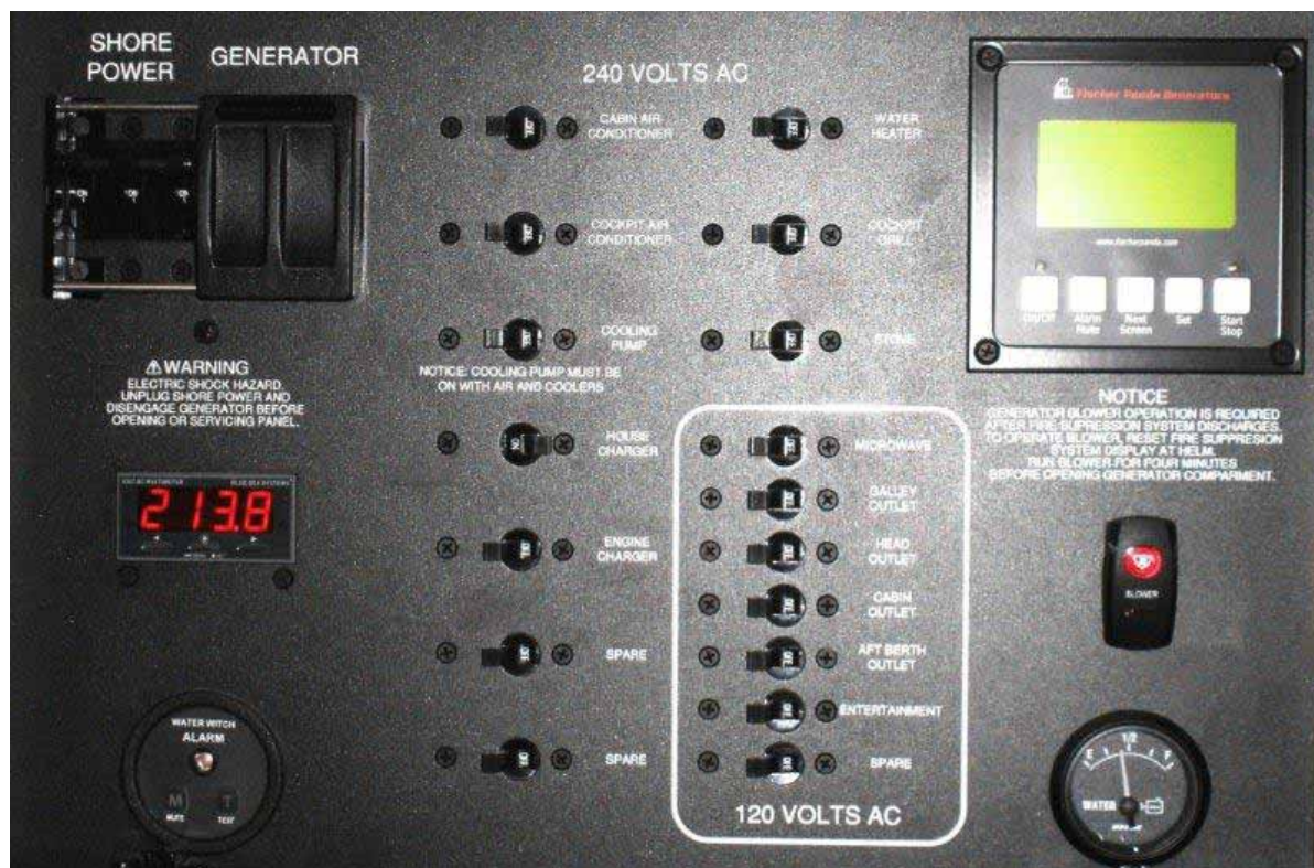
AC Main Distribution Panel (AC MDP)
