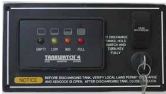
Head Switch Panel
